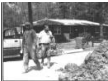
Residents of Larkspur Acres, North Carolina, finish installing a water main in their neighborhood. Their self-help effort enabled the community to affordably bring safe drinking water to their homes.
