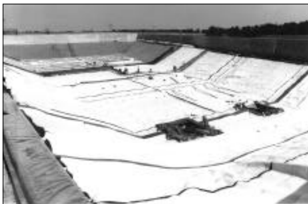
Workers prepare an anaerobic lagoon pretreatment wastewater facility in Jamestown, North Dakota. Financing for the project was arranged by the North Dakota Municipal Bond Bank.
