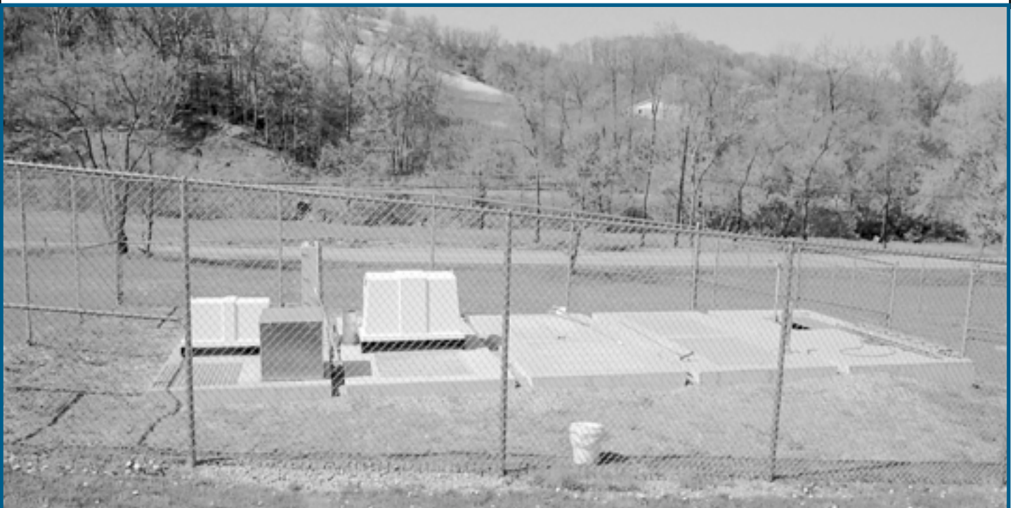
Activated sludge package plant at Mason Dixon Elementary School in Monongalia County, West Virginia.
