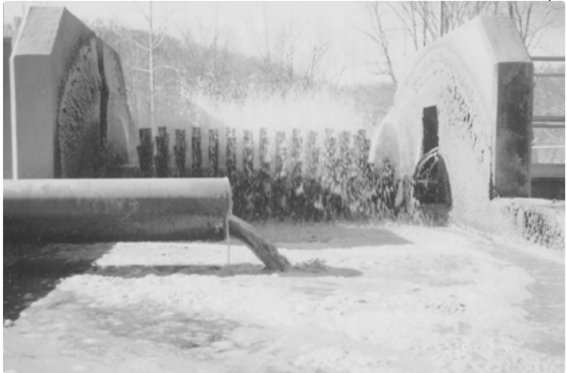
An example of mechanical aeration, provided by rotary brushes, at an oxidation ditch in Jane Lew, WV.
