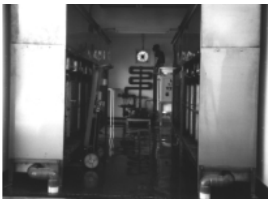
The inside of a trailer-mounted unit. The chemical feed is in the background and the bag units are on either side. (Photo courtesy of Envirodyne Systems, Inc.)
