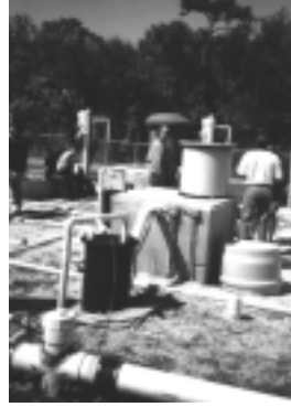
Visitors at the Florida Keys Onsite Wastewater Nutrient Reduction Systems Demonstration Project tour the systems being tested at the Big Pine Key Road Prison in the lower Florida Keys.
