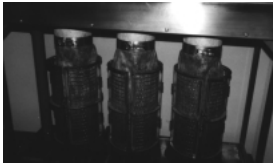
Water is collected in woven, 23-gallon bags. Each bag holds approximately 22.5 pounds of dry biosolids. (Photo courtesy of Envirodyne Systems, Inc.)
