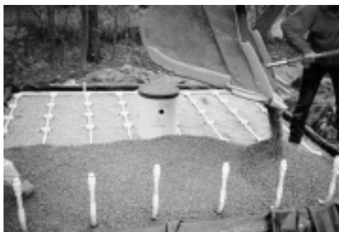
A pre-engineered, pre-packaged intermittent sand filter is installed at a North Gloucester NODP site. (Photo courtesy of Anish Jantrania.)
