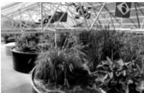
Solar tanks at the South Burlington, VT, municipal sewage treatment system utilize photosynthetic reactions and biological activity to treat 80,000 gpd. (Photo courtesy of Living Technologies Inc., Burlington, VT.)
