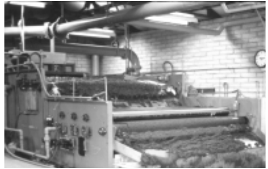
A belt filter press is used in Westminster, Colorado, for solids dewatering. In photo on back cover, biosolids are offloaded to an injector vehicle for land application. (Photos by Dave Cross.)
