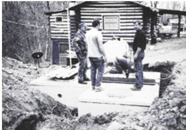
Miracle Mountain's recirculating sand filter system uses two septic tanks (1,000 and 1,500 gallons).
