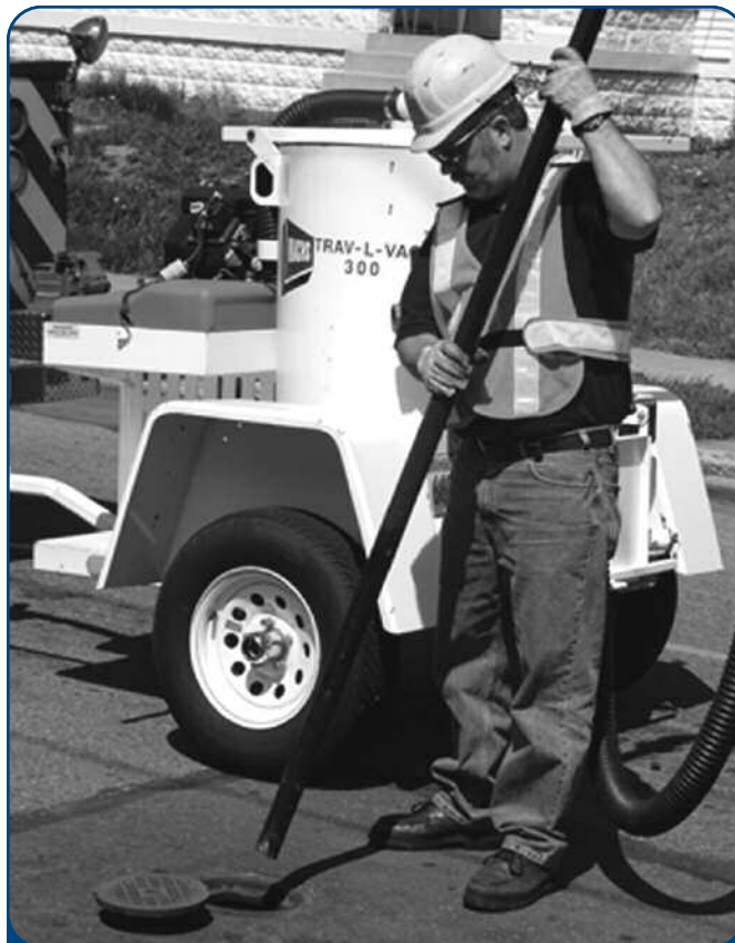
A worker cleans out the valve box with a utility vacuum cleaner. Removing accumulated sediment and dirt from the gate valve curb box must be done before exercising valves.
