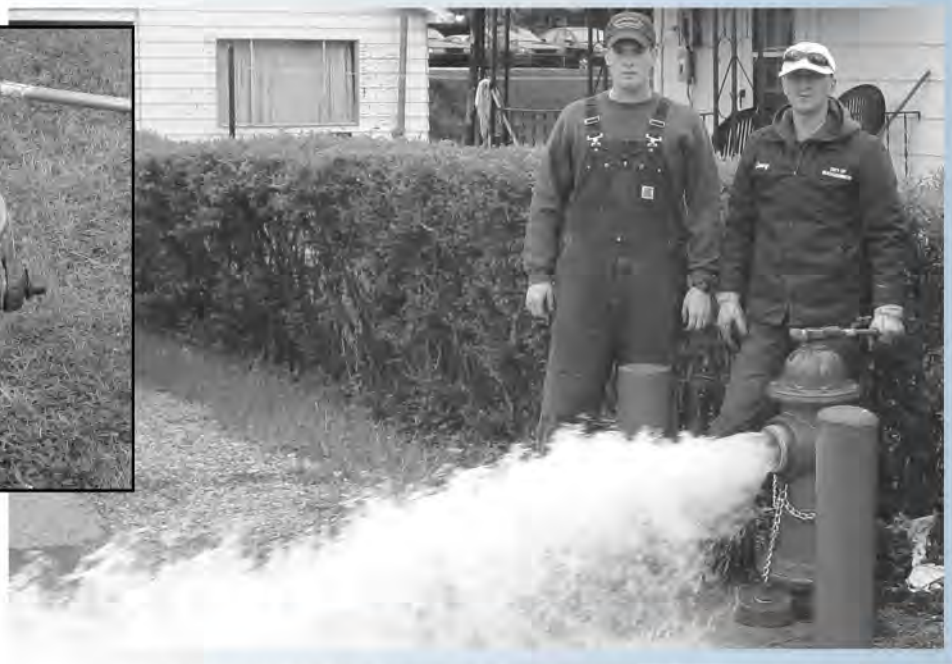
Brian Elmore and Jerry Wamsley of the Buckhannon Water Department in Buckhannon, West Virginia, regularly flush their system's distribution lines.
