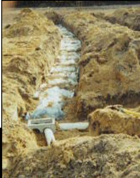
Top: Bottom layer of trench with 6 inches of chips and 4-inch pipe. Middle: Pipe covered with 2 inches of chips. Bottom: Tire chips covered with geotextile material. Job ready for inspection by health department. Photos courtesy of Bob's Septic Tank Company, Waycross, Georgia.
